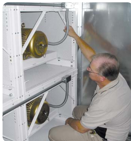
Charles Eversole, the HVAC Manager for the building, initiated the search for a fan system that would provide increased system reliability through fan-unit redundancy.
