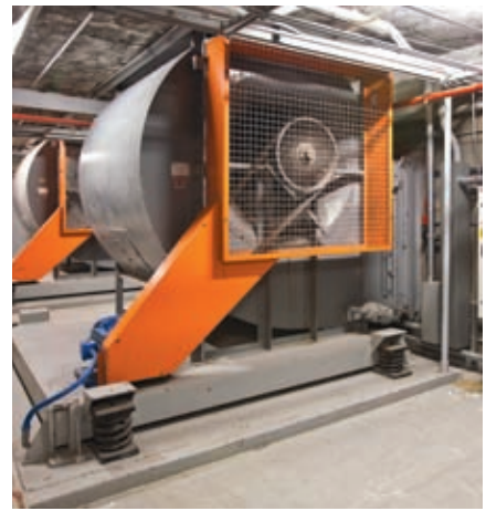
The return fans shown above are reminiscent of the supply fans that were replaced - each the size and weight of a Volkswagon Beetle.
